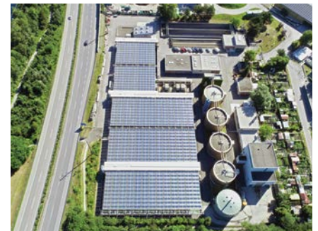
Solarfaltdach ARA Chur (Quelle dhp technology AG) https://dhp-technology.ch/imagefilm-horizon/
